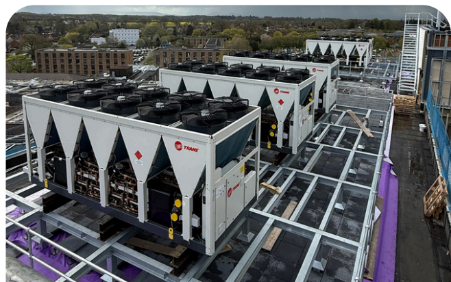
New air source heat pumps now on site
